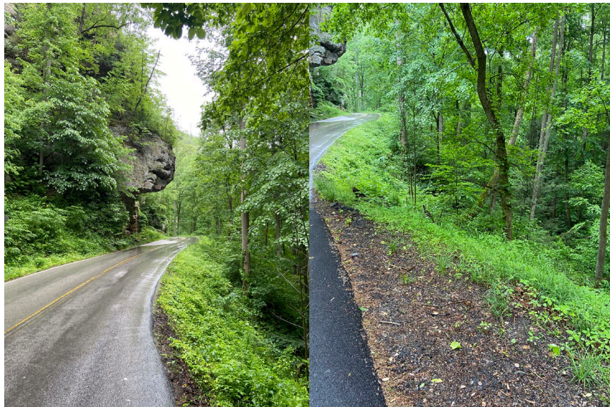
Image 10: Rock overhang exposed on Eastern side of Nada Tunnel. Image 11: Steep fill slope towards Grays Branch on East side of Nada Tunnel.
