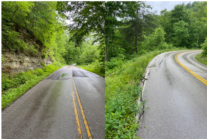
Image 14: Rock cut exposing the Borden Formation with roadway surface repair, MP 0.3.
